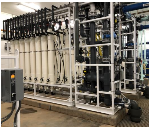
Photo of the new water treatment equipment (membranes) at Selma Water Treatment Plant
