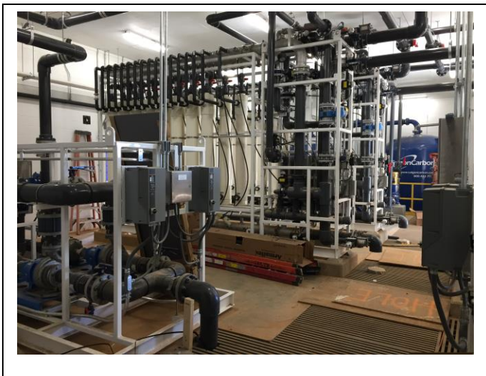
Photo of the new water treatment equipment at Selma Water Treatment Plant
